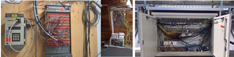
Figure 5. CR7 logger (left) and connection panels 1 and 2.
