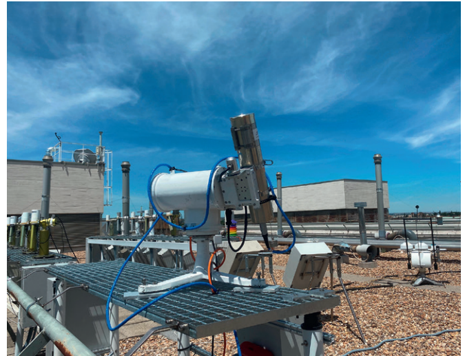
Figure 1. PFR N014 installed at the University of Valladolid (Spain) on 7 June 2022.
