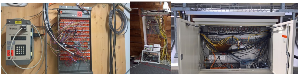
Figure 5. CR7 logger (left) and connection panel 1 and 2
