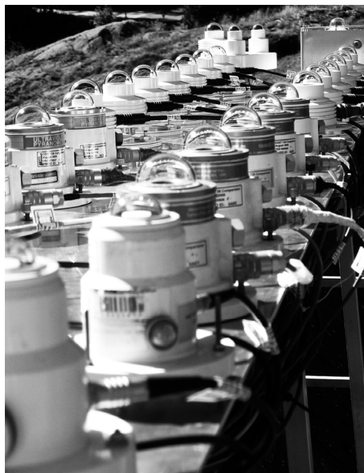
Figure 14. The new platform installed on the roof of the PMOD/WRC with 30 broadband filter radiometers.
